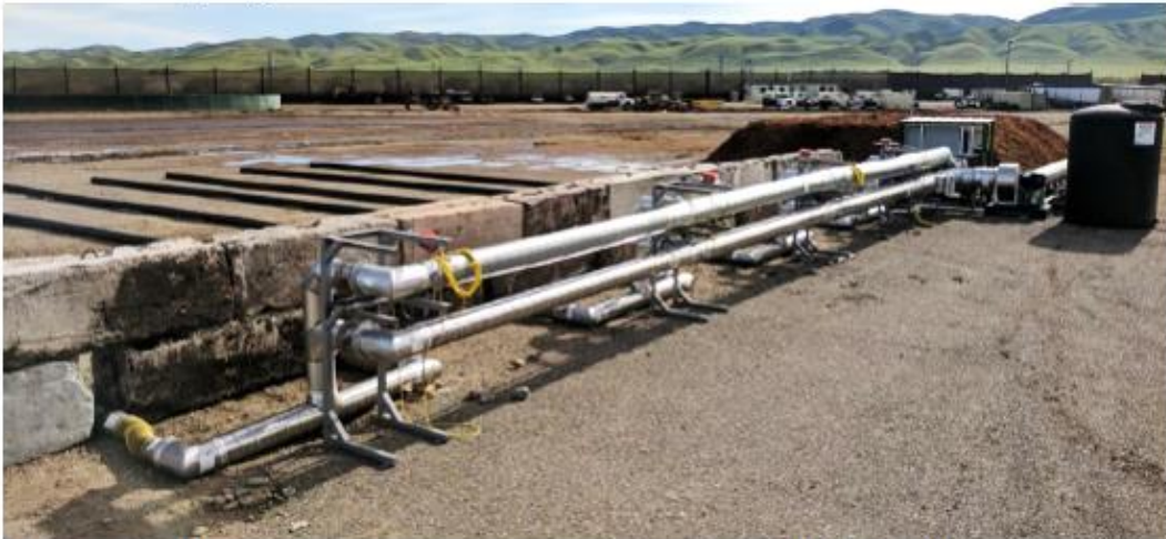
Figure 1. Example of ECS multi aeration mode Pilot CASP System
